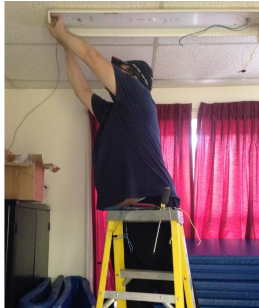
Devin Ingram, replacing the tube lights in a fixture in Grey River.
